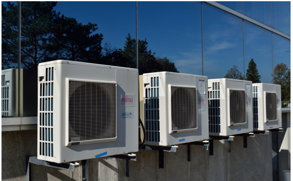
SMPS' in computer systems has increased domestic power quality problems, which damages HVAC components.
