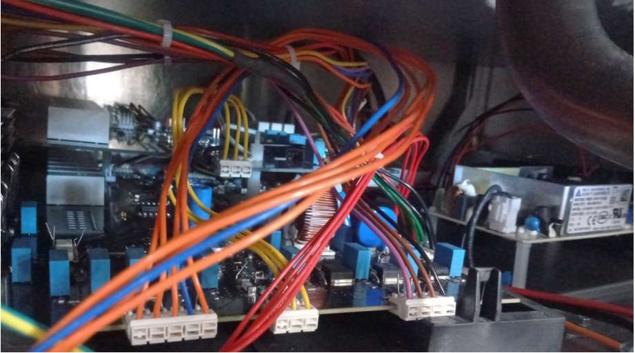
Figure 42 As can be seen, the wiring inside this cabinet was a mess, with 'flying' wires over the PCB, especially over the filter area
