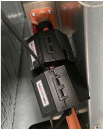
(a) Ferrite cores on cables in the cabinet of a product
