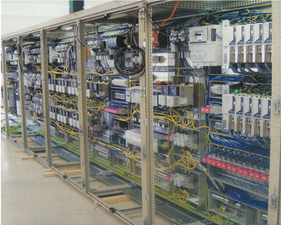
Figure 3: Example of a machine with a number of PDSs Part of a complex installation....
